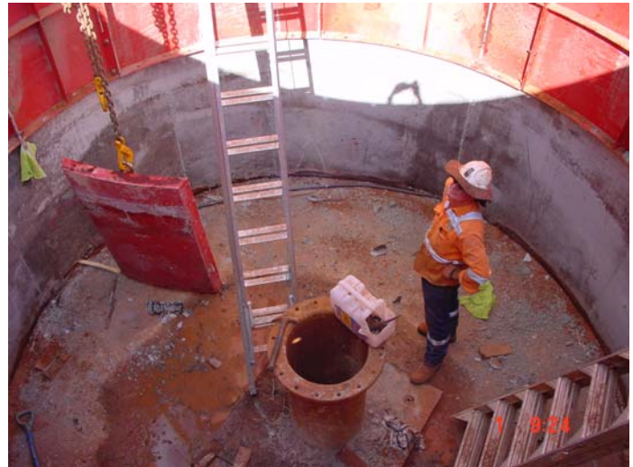
Figure 3: Completing form work of the 4m diameter vent shaft to be raise bored.
